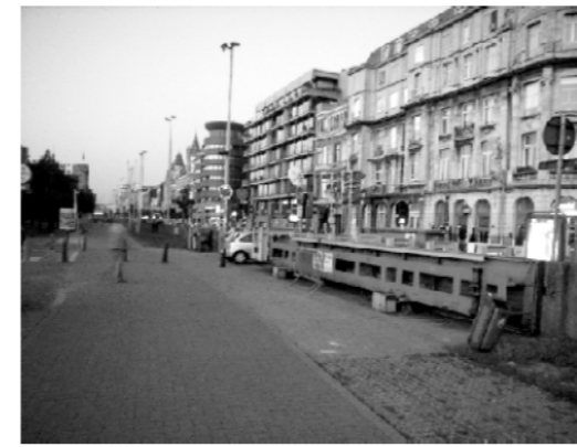
existing mobile protection
